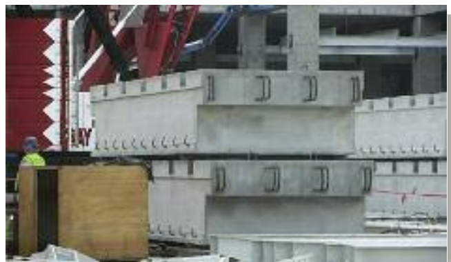
The waffle slabs delivered by Unistress Corporation are enormous, weighing as much as 24 tons each.
