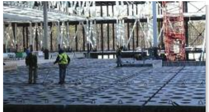
The waffle slabs form the floor of the of the clean room for the new semi-conductor manufacturing facility.
