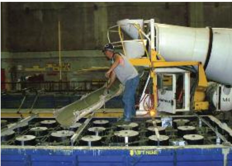
The use of SCC made pouring more efficient and contributed to a better finish.
